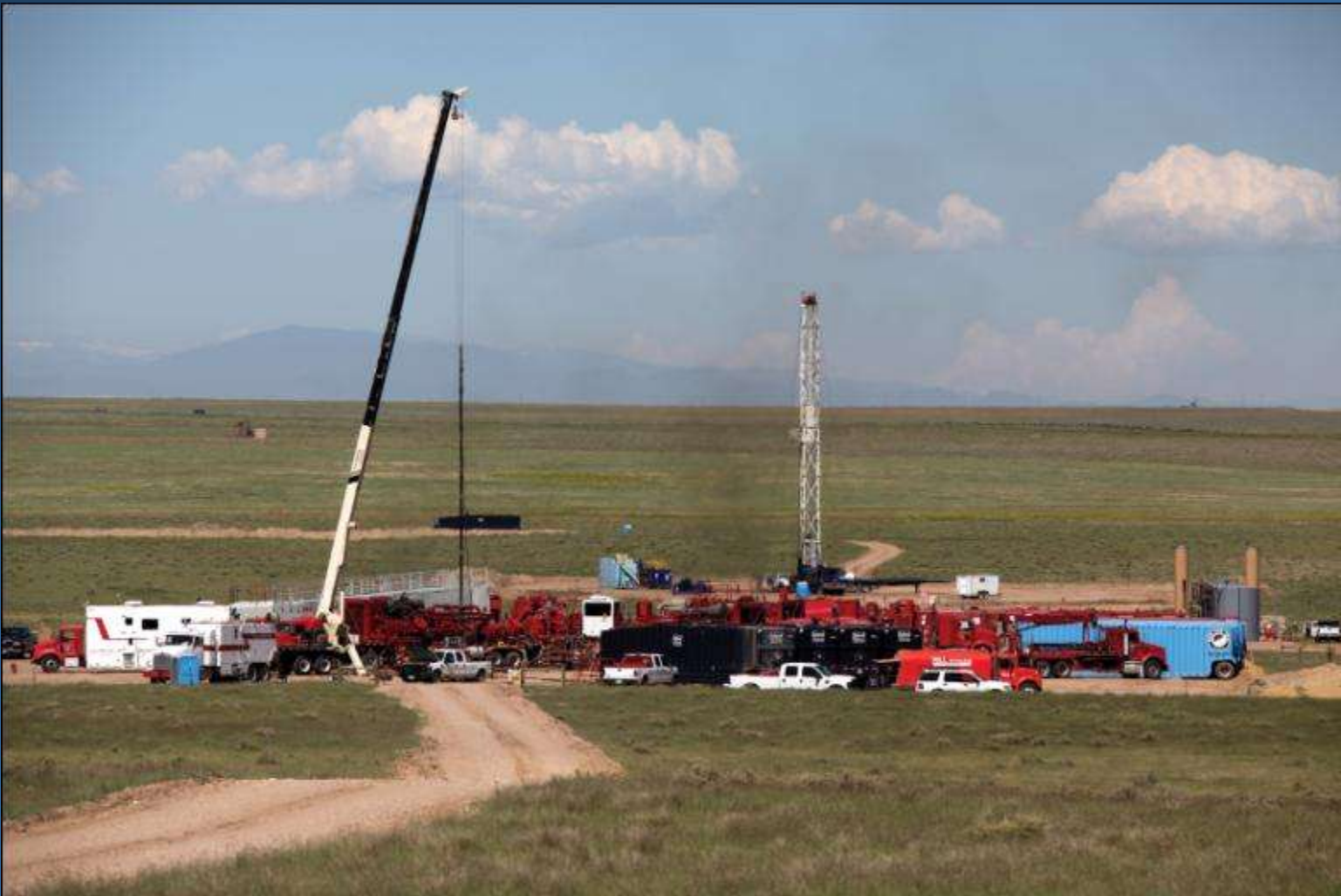
Copyright Hart Energy Publishing. Taken by Lowell Georgia, 2010
